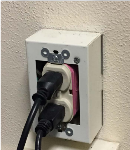
Figure 5 - Receptacle with nylon plate broken off
