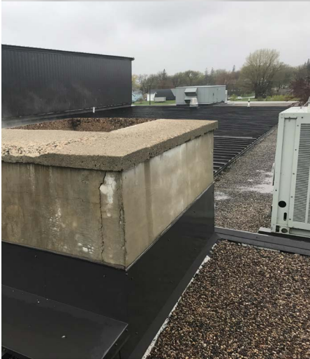
Figure 8 - Damaged cap flashing
