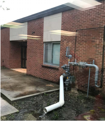
Figure 7 - Pipe on roof drain to direct water away from building
