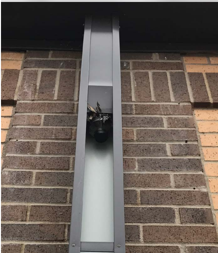
Figure 24 - Blocked roof drain
