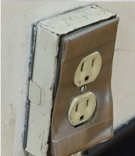
Figure 6 - Damaged receptacle in gymnasium
