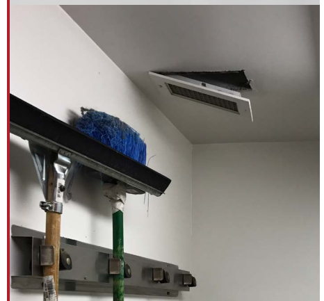
Figure 22 - Exhaust grille falling off
