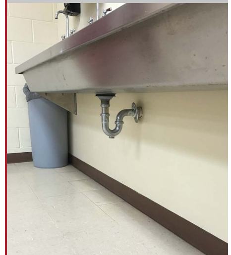
Figure 5 - Missing clay trap in art room
