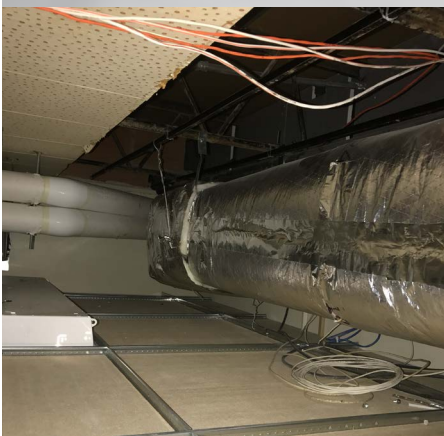
Figure 16 - Loose supply duct insulation
