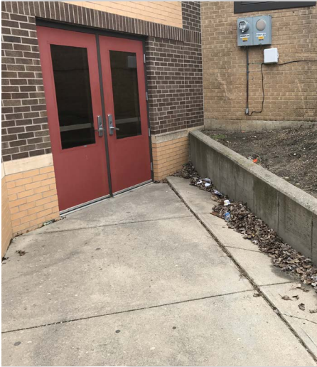
Figure 2 - Tipping sidewalk - suggests movement due to moisture intrusion
