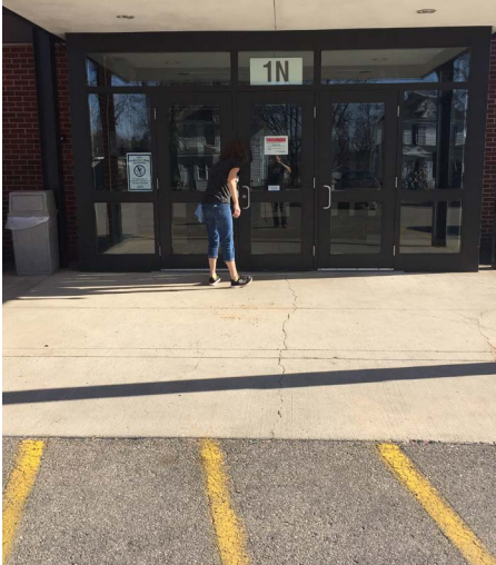
Figure 2 - Cracked sidewalk near door 1N
