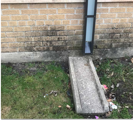
Figure 1 - Area that requires tuckpointing
