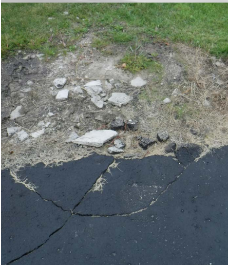
Figure 3 - Cracking bit in south staff lot
