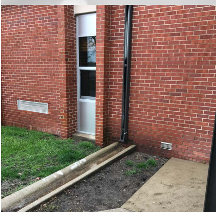
Figure 10 - Leaking abandoned louver
