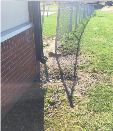
Figure 8 - Playground fence and erosion
