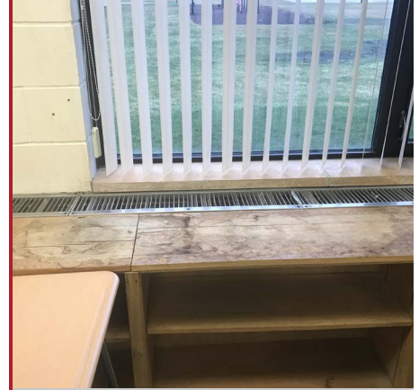
Figure 10 - Evidence of water damage to casework
