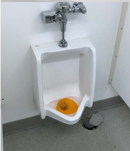
Figure 9 - Broken floor cleanout cover
