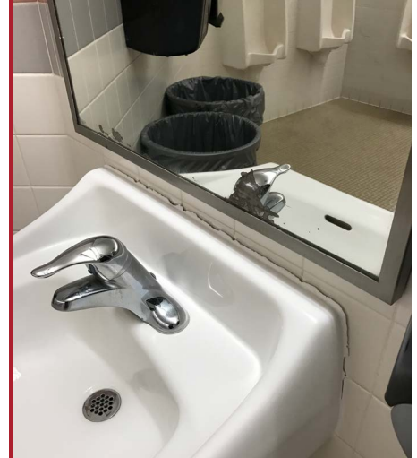
Figure 10 - Missing aerator on faucets
