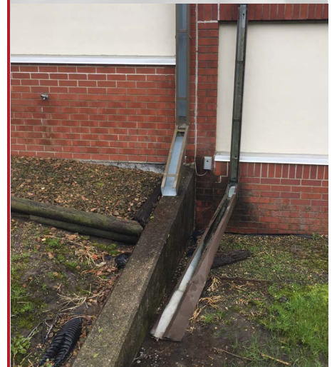
Figure 6 - Poor storm drainage management
