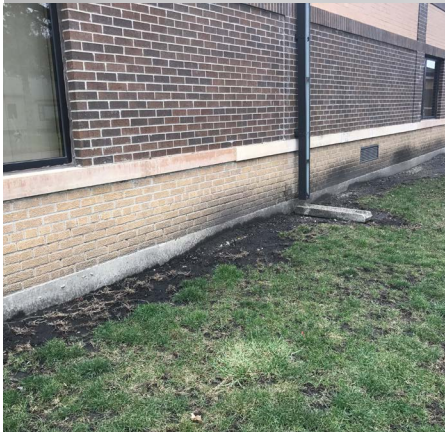
Figure 2 - Area that requires tuckpointing
