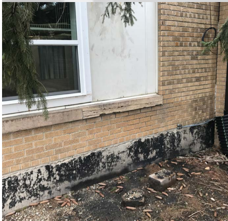
Figure 4 - Area that requires tuckpointing, sealants, or new walls
