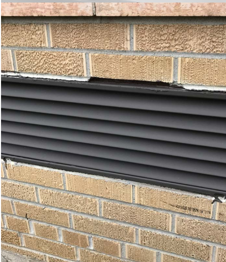
Figure 25 - Bad louver seals
