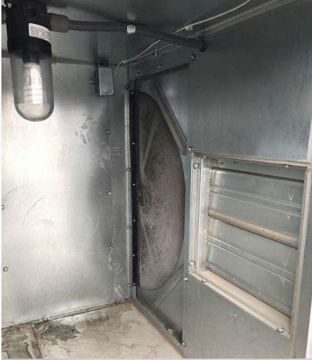
Figure 23 - Dirty energy recovery wheel
