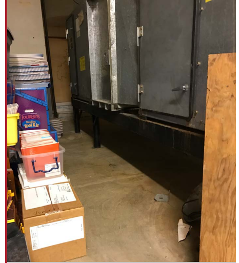
Figure 4 - No vibration isolation on AHU
