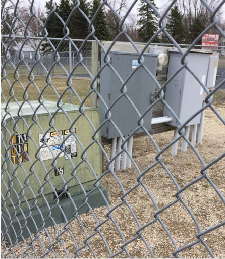
Figure 4 - Football field electrical backboard
