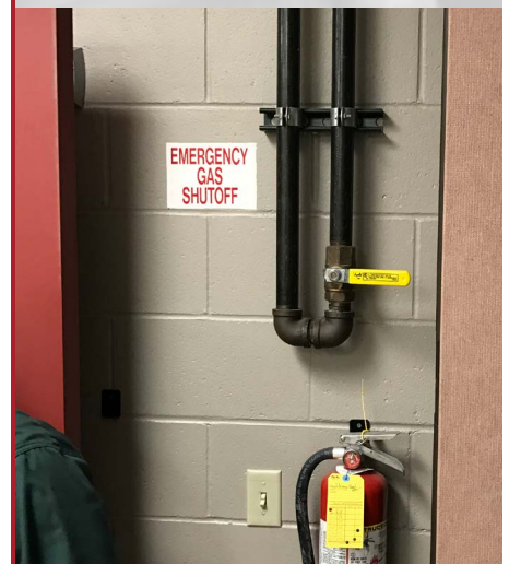
Figure 6 - Missing emergency gas shut-off button
