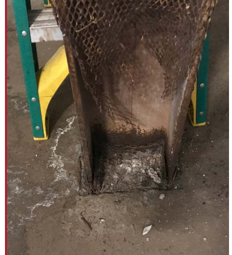
Figure 5 - Rusted and degraded column base plate in boiler room
