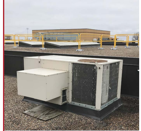
Figure 11 - Damaged condenser fins on RTU
