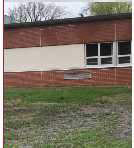
Figure 3 - White streaks in the brick which indicate previous tuckpointing attempts
