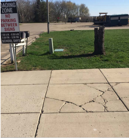
Figure 1 - Cracked sidewalk near loading sign
