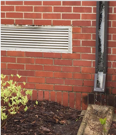
Figure 2 - Grille that could be removed
