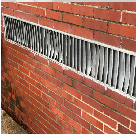
Figure 9 - Damaged intake louver
