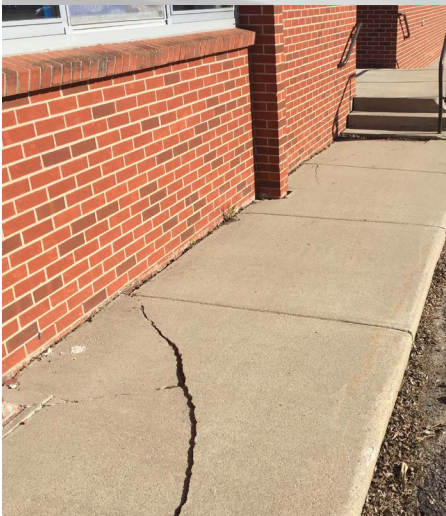
Figure 3 - Cracked sidewalk near door 6S
