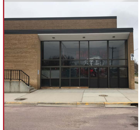
Figure 7 - Windows with seal failure and rusted frames
