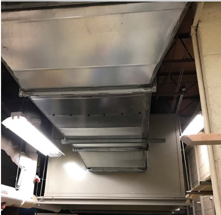
Figure 8 - No spring vibration isolation present on AHU
