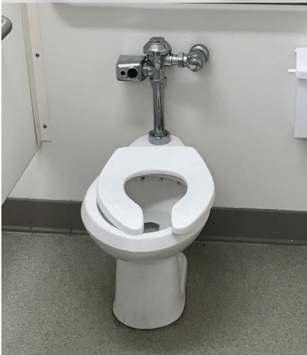
Figure 8 - Broken toilet seat
