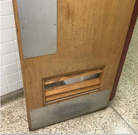
Figure 6 - Damaged air grill in door
