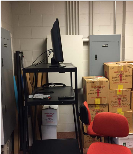
Figure 5 - Electrical panels without proper clearances maintained
