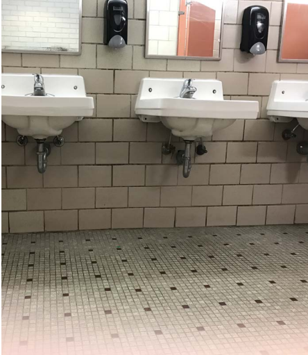
Figure 1 - Restroom sinks which do not meet current ADA standards
