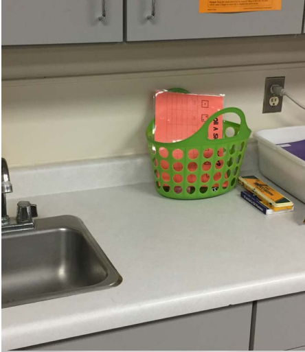
Figure 4 - Non-GFCI receptacle near sink
