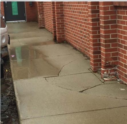
Figure 4 - Cracks in sidewalk
