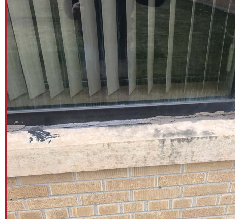
Figure 5 - Poor sealants around window frames
