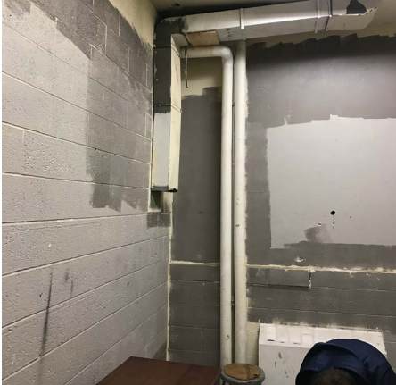
Figure 7 - Improper exhaust flow in paint room
