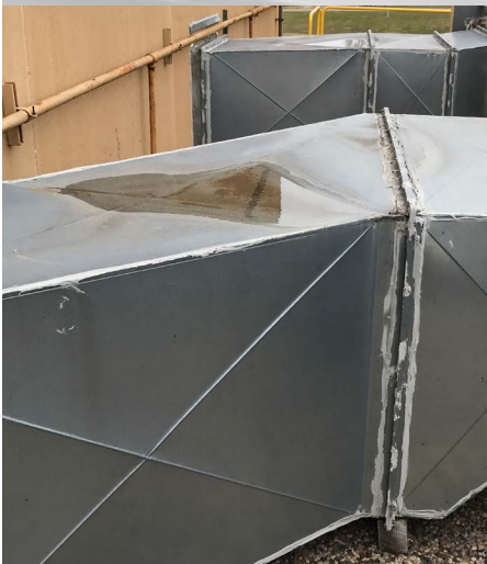
Figure 3 - Exterior ductwork not sloped properly
