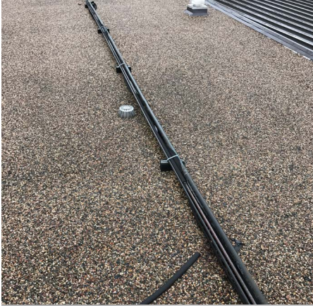
Figure 7 - Missing insulation on refrigerant lines
