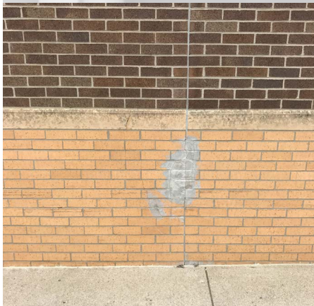
Figure 3 - Area that requires tuckpointing, sealants, or new walls
