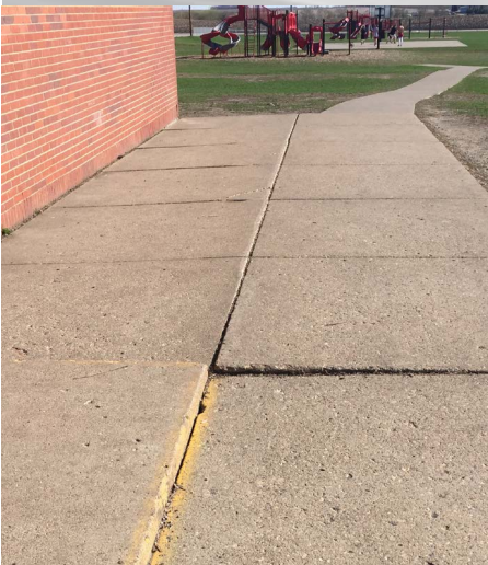
Figure 6 - Sidewalk settlement due to inadequately-compacted backfill
