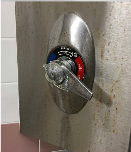
Figure 3 - Leaking shower faucet
