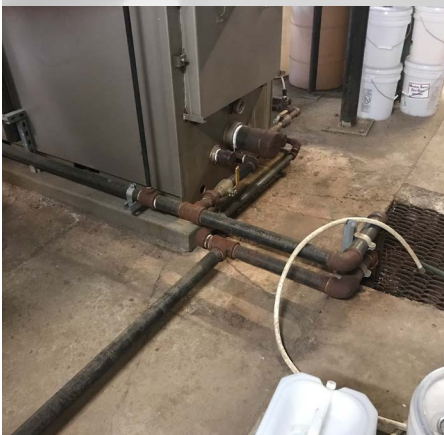
Figure 4 - Boiler room piping, creating a trip hazard
