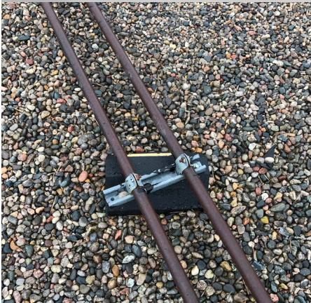
Figure 8 - Broken gas pipe supports
