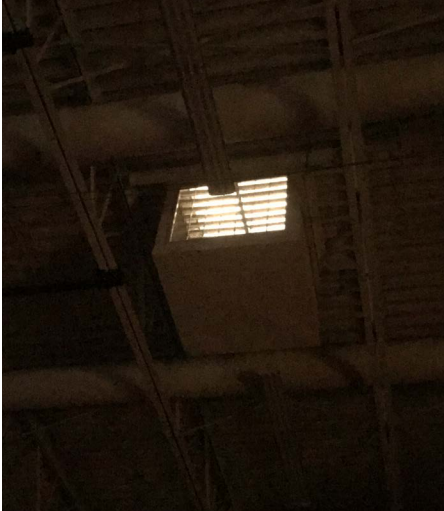
Figure 1 - Gym relief dampers stuck open
