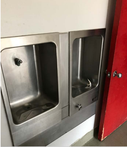
Figure 7 - Broken drinking fountain
