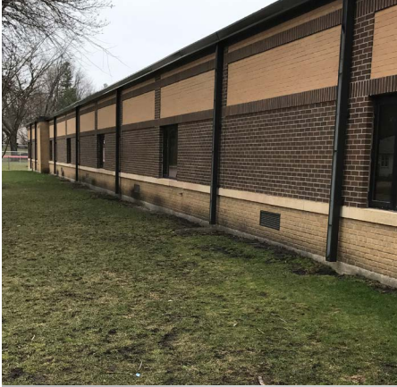
Figure 15 - Louvers low to ground
