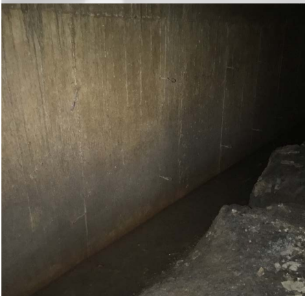
Figure 10 - Standing water in area C crawl space
