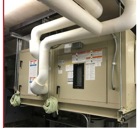
Figure 19 - Missing vibration isolation
