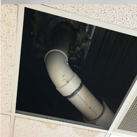
Figure 5 - Uninsulated roof drain
