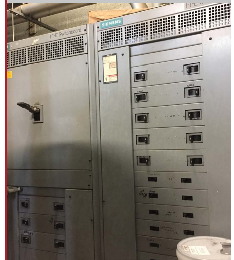
Figure 2 - Main electrical gear
