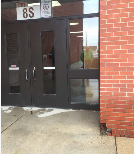
Figure 1 - Damaged/missing bricks at corner
