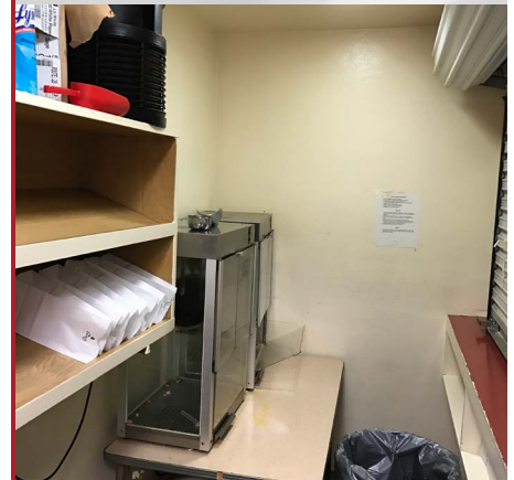
Figure 13 - Exhaust air missing in concession stand
