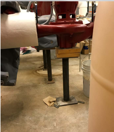
Figure 3 - No vibration isolation on pumps
