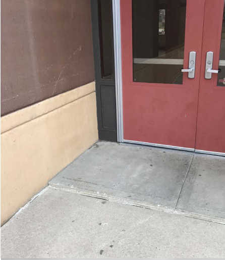
Figure 1 - Lip in concrete
