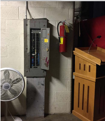
Figure 6 - Older electrical panel
