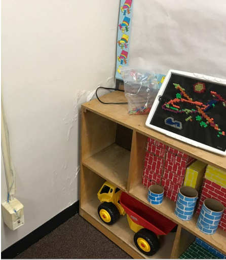
Figure 4 - Damage adjacent to casework
