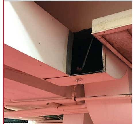
Figure 14 - Missing ductwork in wrestling room
