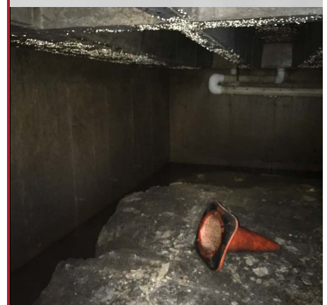
Figure 13 - Crawlspace with moisture concerns
