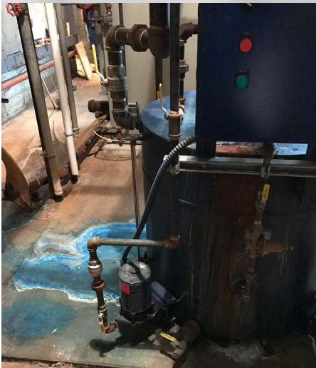
Figure 2 - Leaking boiler feed unit
