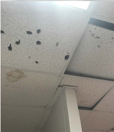
Figure 2 - Damaged ceiling in need of replacement
