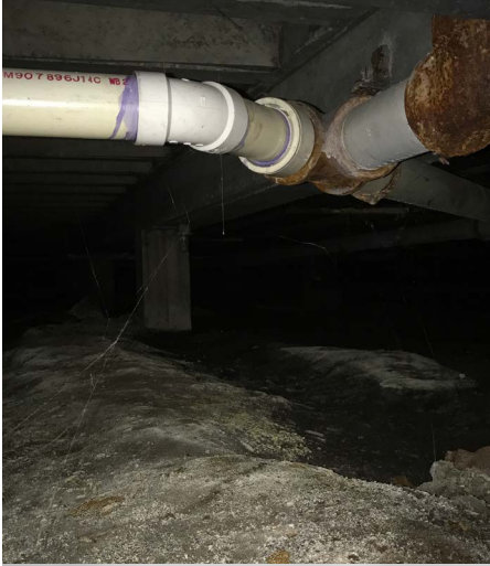
Figure 14 - Moisture concerns in unexcavated area
