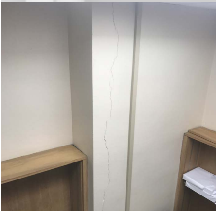
Figure 3 - Wall crack on masonry column
