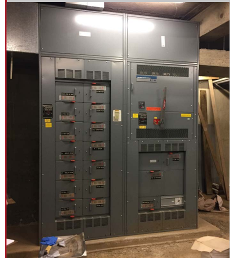
Figure 2 - Main electrical gear
