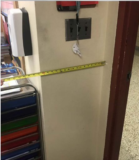
Figure 3 - Large wall depth, which is not ADA-compliant
