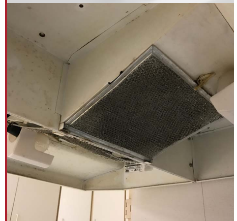
Figure 21 - Stovetop hood with no airflow
