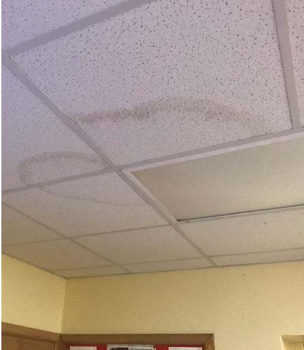
Figure 1 - Discolored ceiling tiles
