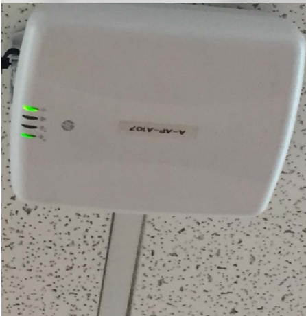
Figure 2 - Typical wireless access point
