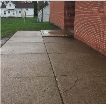
Figure 3 - Cracked sidewalk and 1-inch lip at sidewalk edge, creating accessibility issues
