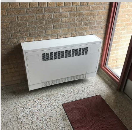
Figure 17 - CUH in vestibule in area C not working
