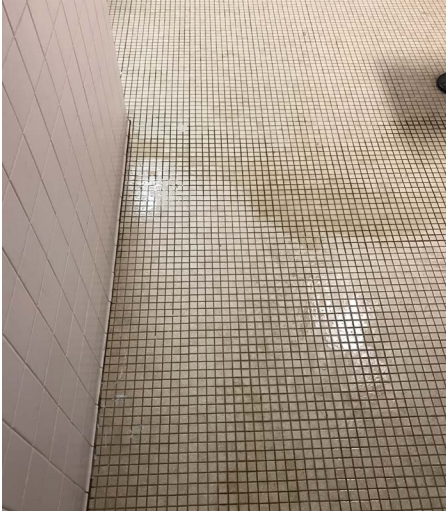
Figure 1 - Water coming through wall
