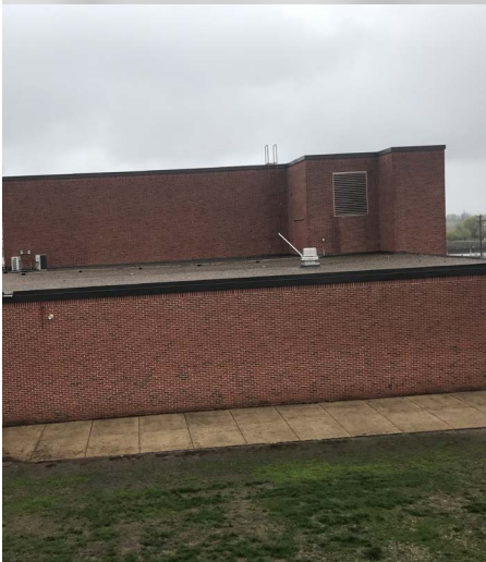
Figure 5 - Extended plumbing roof vent
