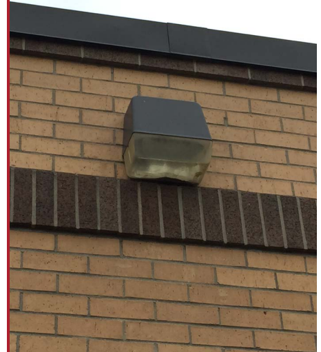
Figure 7 - Existing exterior HID light
