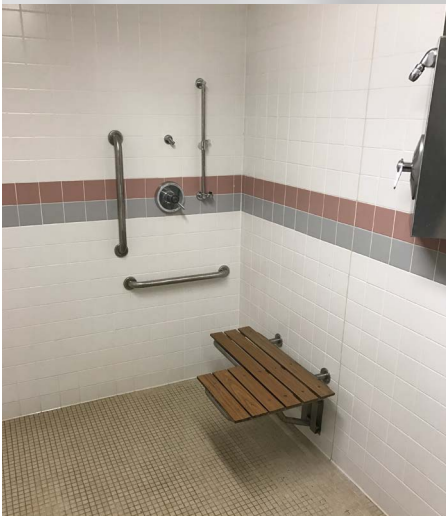
Figure 2 - Broken ADA shower
