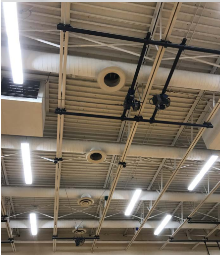
Figure 2 - Broken diffusers in gymnasium
