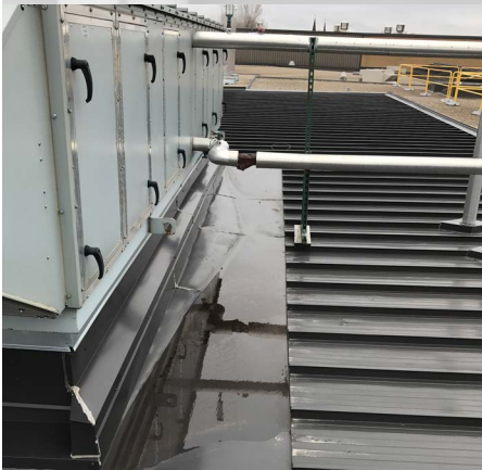
Figure 9 - Improper crickets around the RTU
