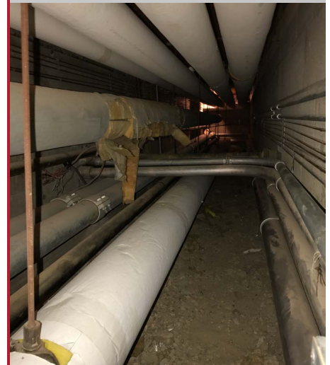
Figure 5 - Insulation falling off in tunnels
