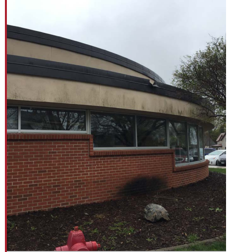
Figure 4 - EFIS surface in need of cleaning
