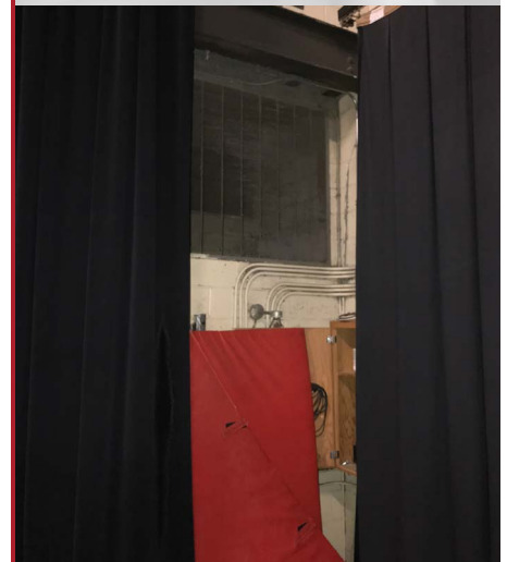
Figure 13 - Space lacking air return
