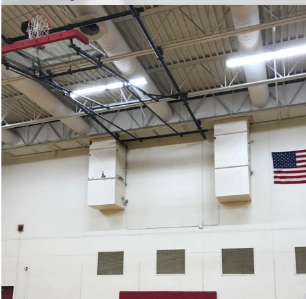
Figure 18 - Paint coming off ductwork
