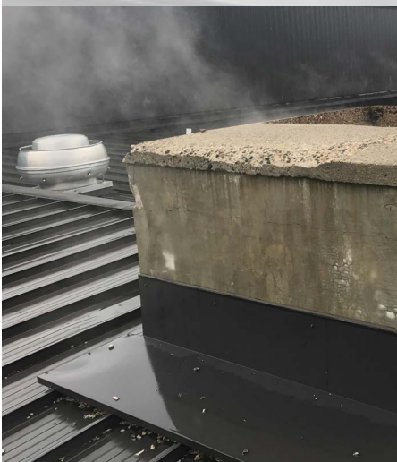
Figure 9 - Damaged Cap flashing
