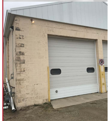
Figure 3 - Exterior paint peeling
