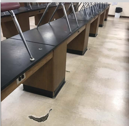
Figure 9 - Damaged floor in science area
