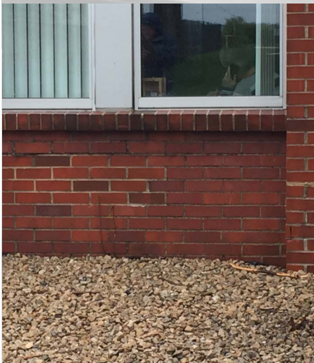
Figure 3 - Area in need of tuckpointing
